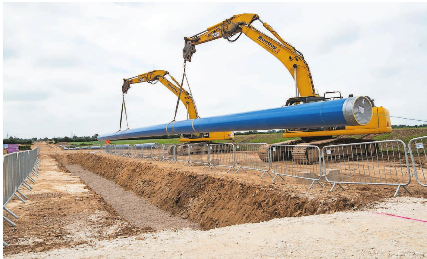
Anglian Water has started to lay the pipeline in Lincolnshire. It will bring water to Suffolk and Essex from the wetter parts of north Lincolnshire
